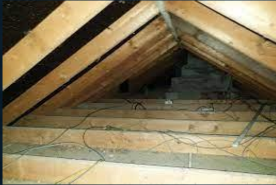
Inadequate or poorly fitted insulation
